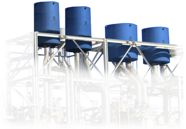
Vent Silencer Array at a Power Plant
